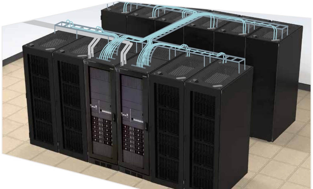
Figure 3a: 140kW initial deployment Two DC UPS modules power blade server racks
