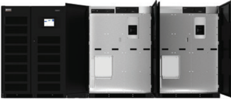
Liebert® battery cabinet with Albér BDSi Battery Monitor. First battery cabinet (center) with Controller and DCM/LM. Additional battery cabinet (right) with DCM/LM only.
