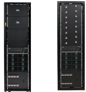
Power Module/Bay with Bulk Distribution Panels (left) with Load Distribution Panel (right)
