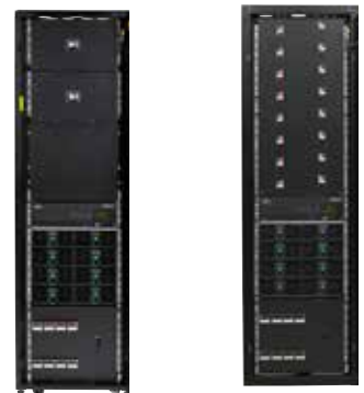
Power Module/Bay with Bulk Distribution Panels (left) with Load Distribution Panel (right)
