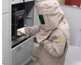
Arc Flash / Power System Engineering
