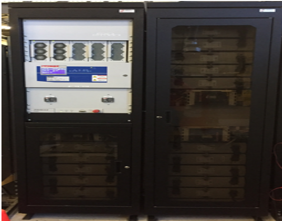
Figure 2. Li- ion installation
