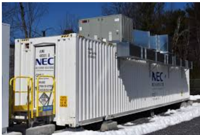
Figure 1 – NEC's Lithium ion Battery Energy Storage System Installed in Sterling, MA
