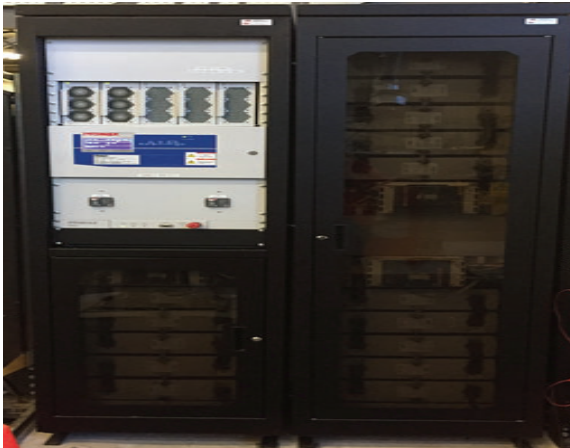
Figure 2. Li- ion installation
