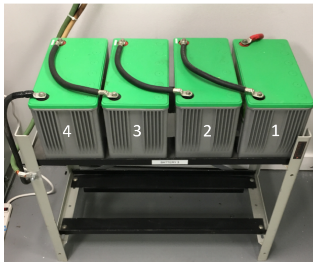
Figure 13. Properly Numbered 4 Unit, 48V Battery Using 12V Multicell Units.
