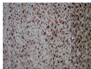
Dirt and incorrect distribution
