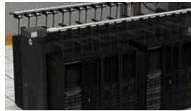
IDC data rooms in finance, telecom, government and IT industries
