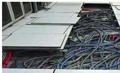
Typical Data Center with Power Cables and Conduit
