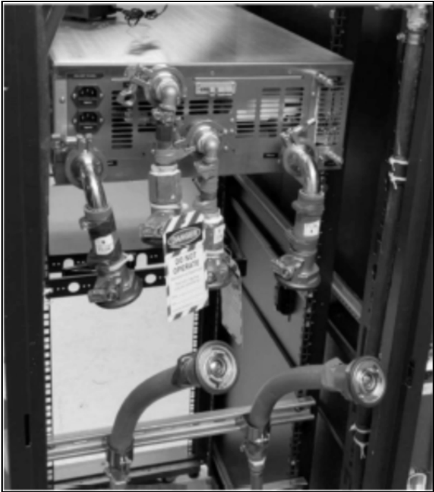
Figure 5.6 Unit in Rack
