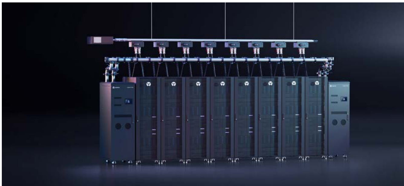
Liquid-cooled row supported by Vertiv™ CoolChip CDU and Vertiv™ CoolChip Fluid Network
