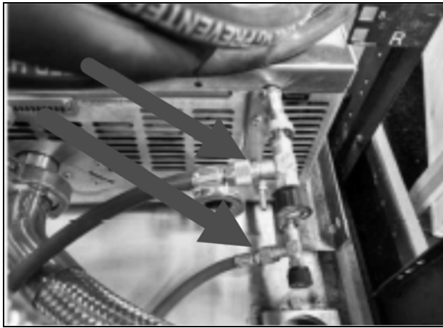
Figure 5.2 End in External Containment
