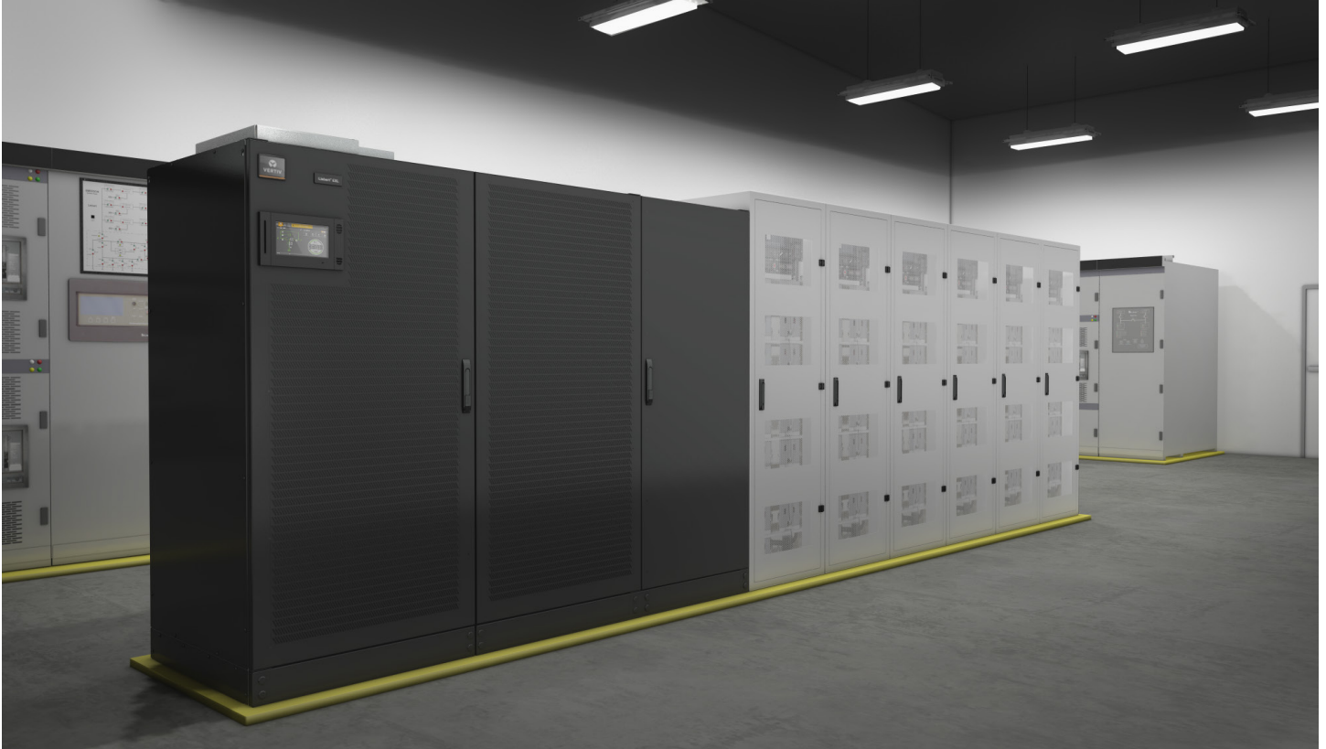
Lithium-ion Battery cabinets sit next to a 1200kW UPS
