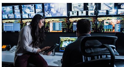
Process control rooms
