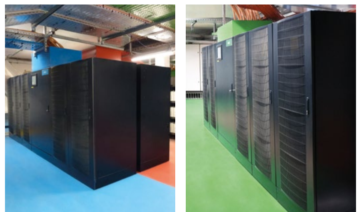
Liebert Trinergy UPS installed in a 3 x 2(N+1) redundancy configuration
