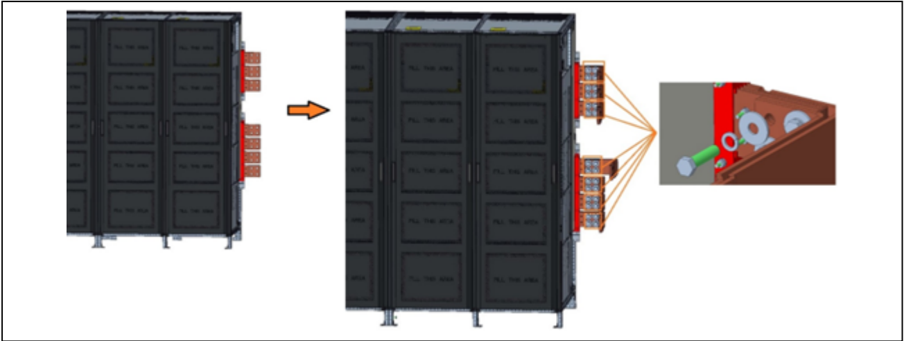
Figure 3.29 Front Side View, Final Installation of Copper Bars from STS to Cores
