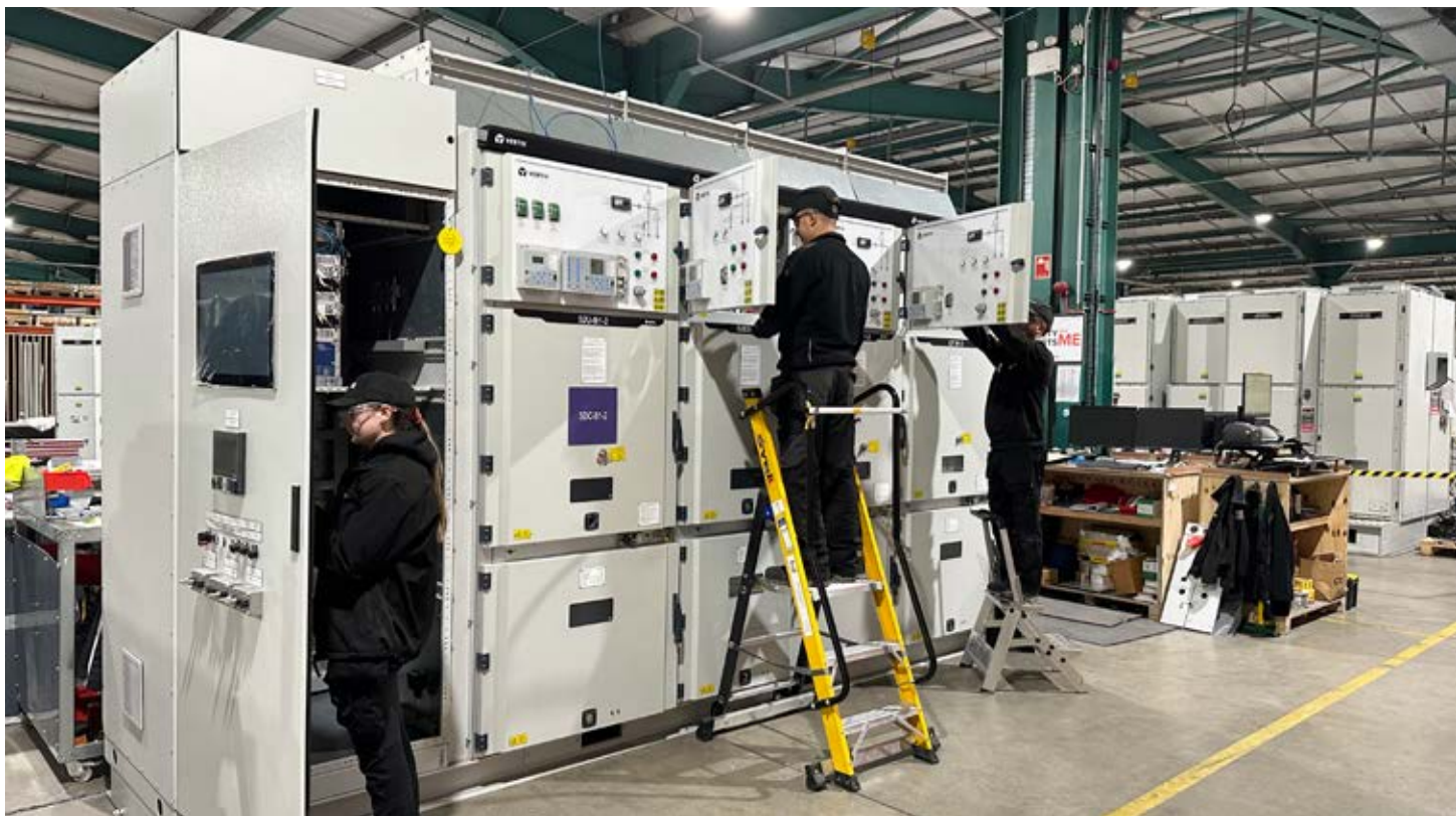
Switchgear assembling by our Vertiv apprentices.
