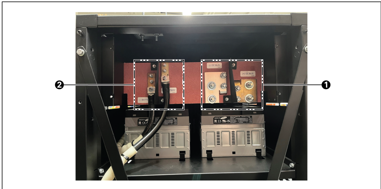
Figure 5.5 Battery Cabinet DC Cables—Voltage Check
