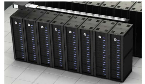
Data Center with Liebert® MBX
