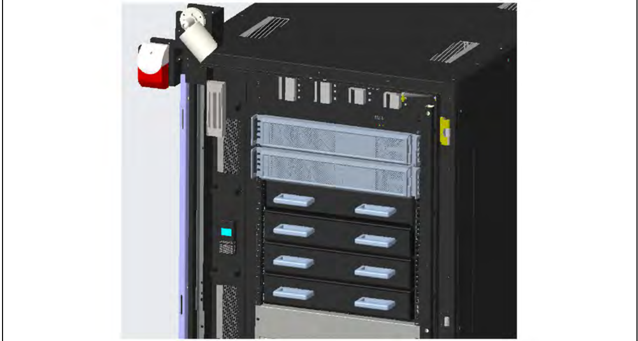
Figure 4.13 Installed Position of Battery Module
