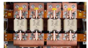
Battery / Load Connection Unit
