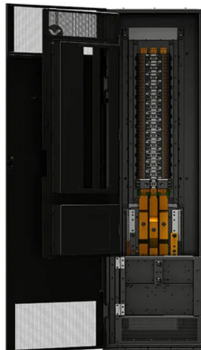
Vertiv™ Panel with Breakers
