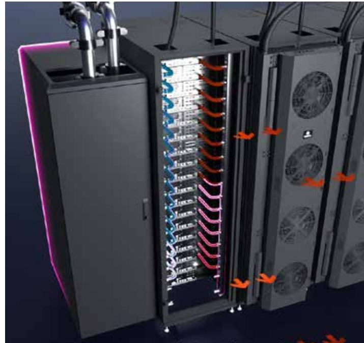
AI GPU Server (Liquid Cooled) Rack Manifolds | Row Coolant Distribution Unit
