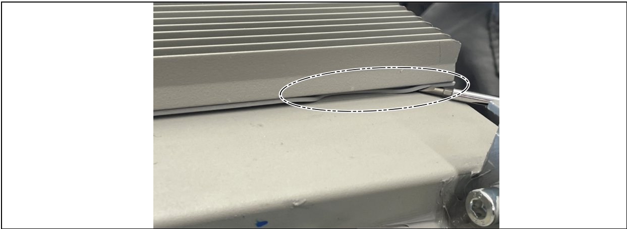
Figure 6.10 Example of Partially Dislodged Gasket
