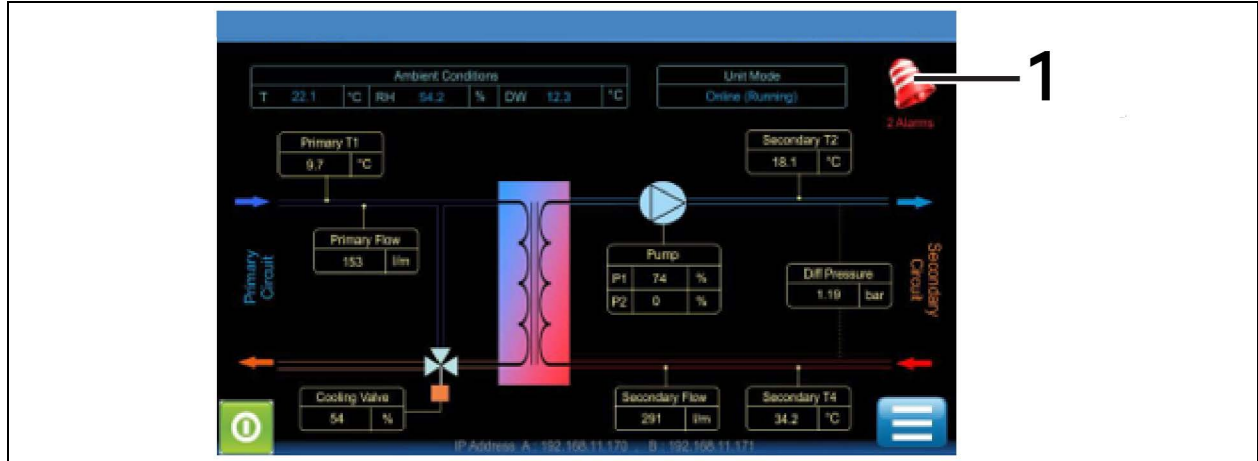
Figure 4.16 Control Screen Alarm Indication
