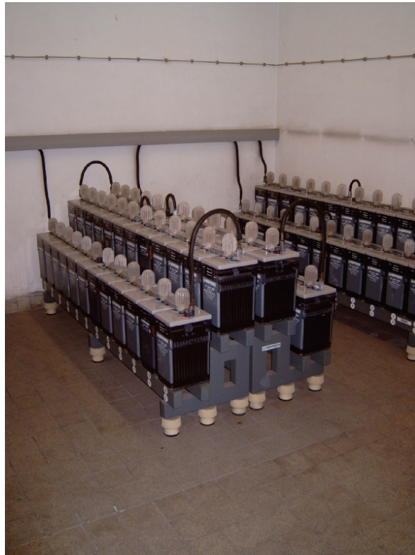
Fig. 10 - RWE Mülheim / electric power transformation substation for steel mill (installed 20.04.1984 / replaced 2007)
