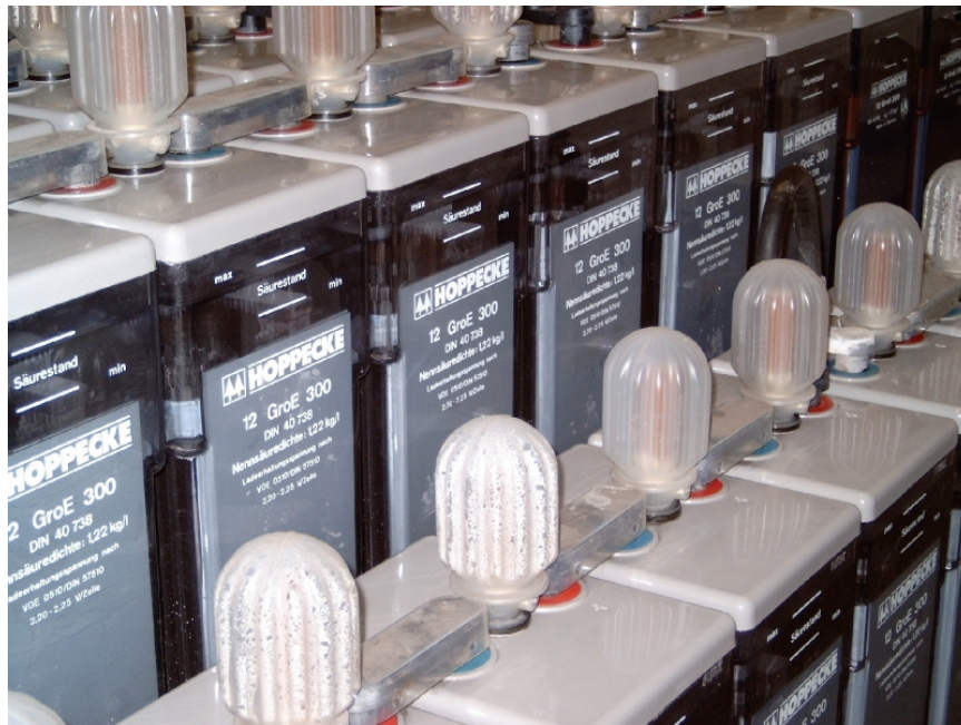
Fig. 9 – With proper design the catalysts can reach an age of more than 20 years (units installed in 1984)
