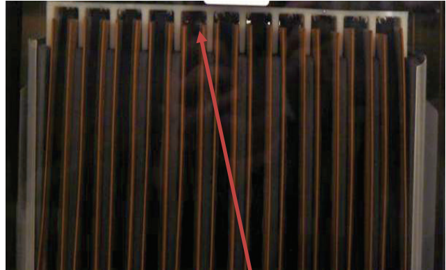
Figure 17. Incorrect insulated plate supports.
