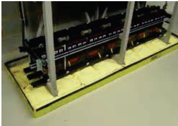
Figure 23. Spill containment system.
