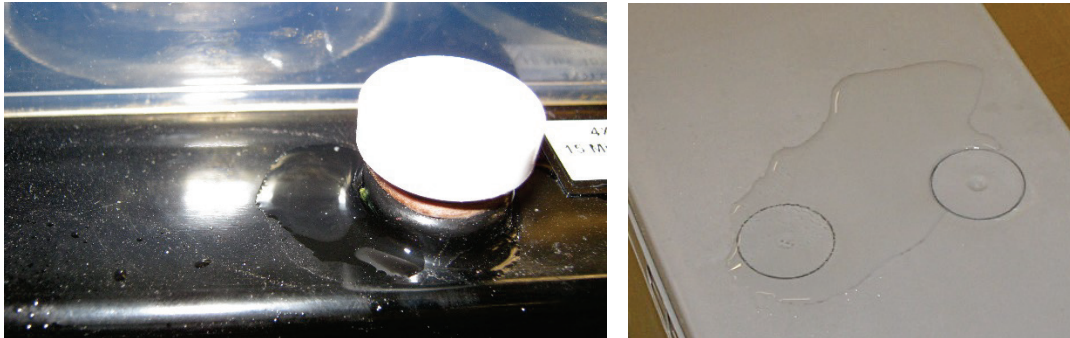
Figure 5. Electrolyte or Water on Top of Battery Container.
