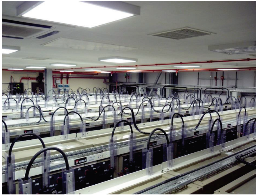
Figure 7. Battery Room at Lerwick Power Station
