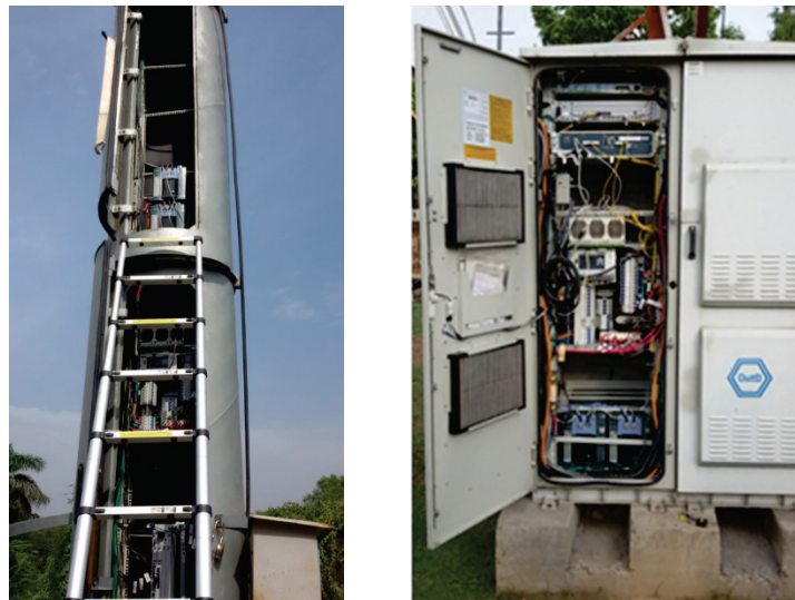
Figure 5: GBM (left) and outdoor cabinet (right) with NCA Li-ion batteries (Courtesy: Reliance Jio Infocomm Limited)
