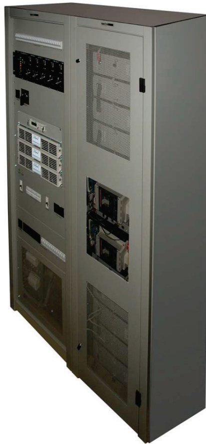
Figure 9: Compact Power Center (7 kW for 2 hours) Courtesy: Southern Company
