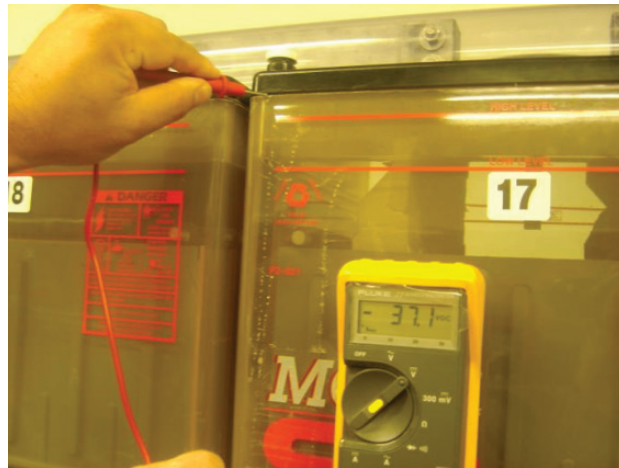
Figure 4. A leaking jar-to-cover seal could become the energy source that results in a battery fire.
