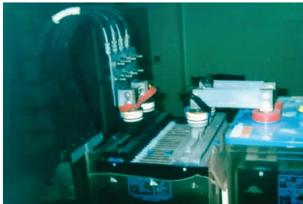
Figure 3. A 3,900 AH cell exploded when an electrostatic discharge as a result of a technician's errors.
