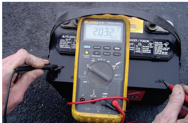
Figure 7. As is seen, there is a two (2) volt loss across the top of the cover as a result of electrolyte leakage.
