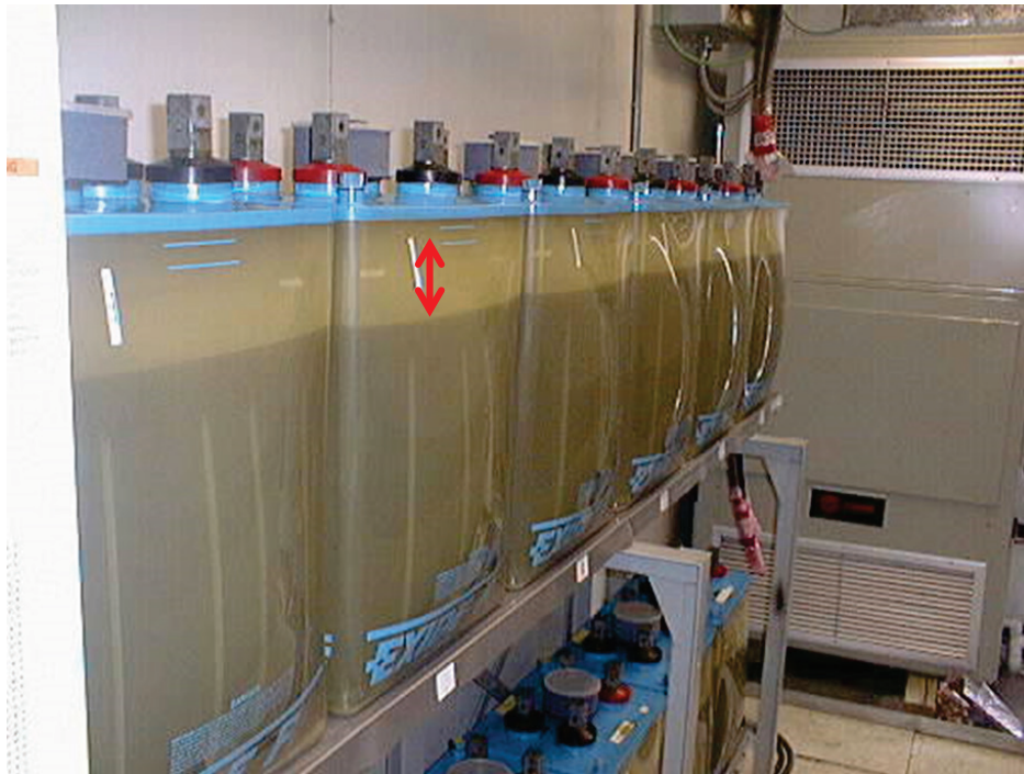
Figure 1. Lead calcium battery cells with jars that bulged due to an overheating condition in the wake of an HVAC system failure. Note the drastic electrolyte level drop (Arrows) that resulted from jar bulging.
