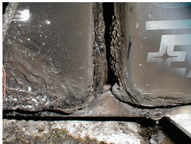
Figure 5. A leaking jar resulted in fire to spill containment bags beneath a battery.
