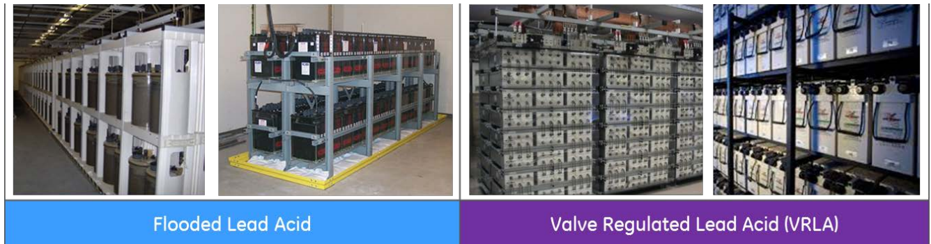
Figure 2 - Lead Acid Batteries in Telecom applications
