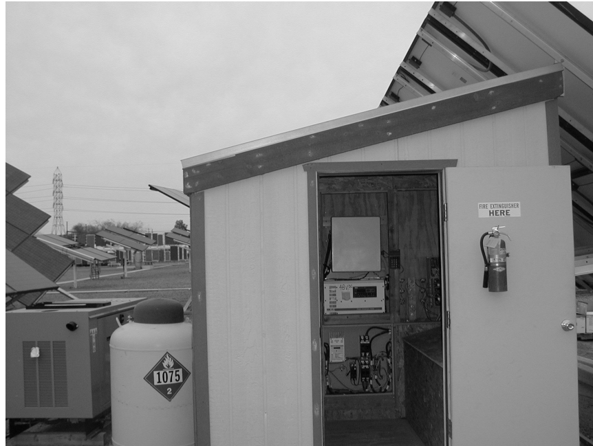
Figure 3: Remote Residential Electric Test System used for Demonstration of Alternative Configuration Unit
