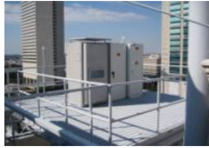
Rooftop application, L to R, BTS radio cabinet, PEM fuel cell cabinet, H2 fuel cabinet.
