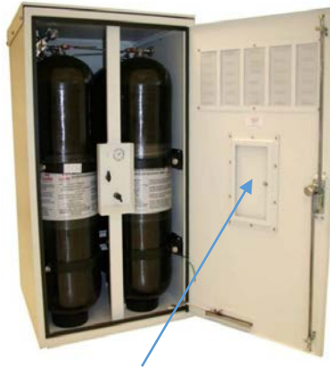
Fuel Cabinet FIP Port, with Small Access Door
