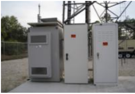
Ground level application, L to R, BTS radio cabinet, PEM fuel cell cabinet, H2 fuel cabinet.
