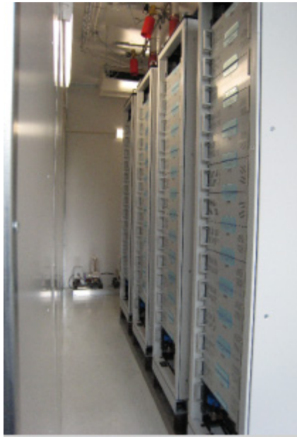
Figure 6. 5200 V lithium-ion battery for grid support
