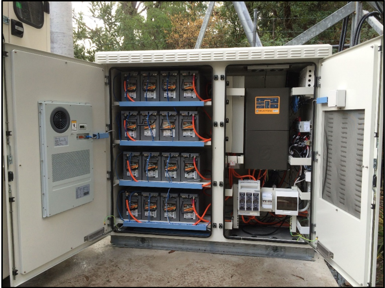
Figure 8. Cabinet showing battery installation
