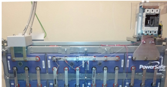
Figure 3. Disconnect Terminated on Negative Pole
