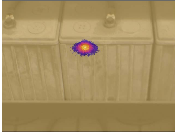
Figure 3. A blended thermal image of a VRLA jar on a float charge in a stationary power application
