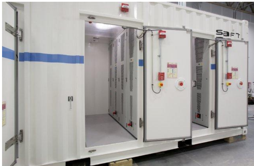
Figure 3. Containerized Li-ion energy storage system
