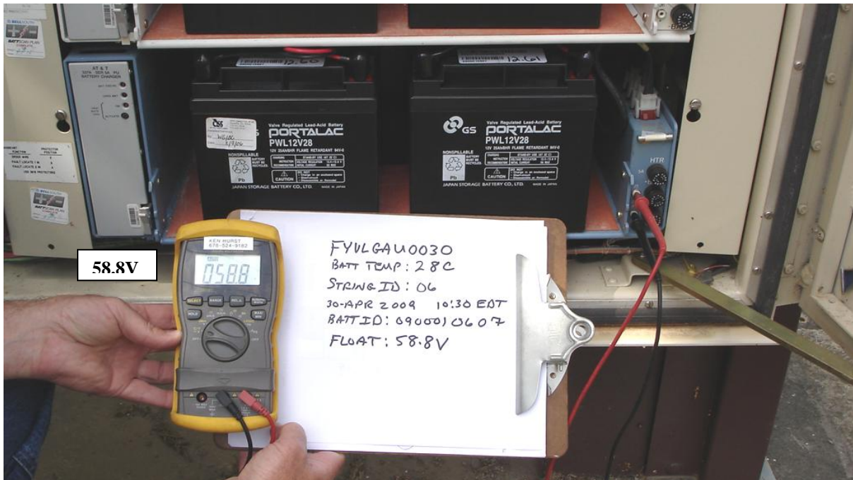
Figure 2. Without the SCD-100 Installed at FYVLGAU0030 – 58.8VDC @ 28C
