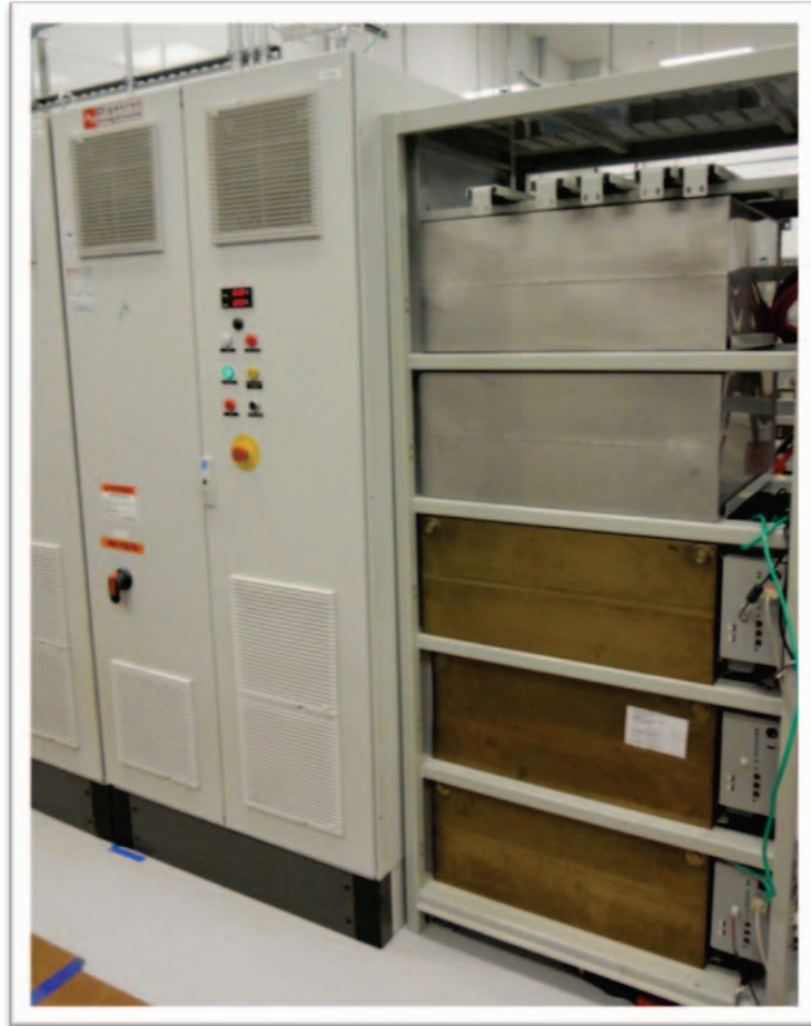
Figure 3: Three-battery test system at GE Energy Storage
